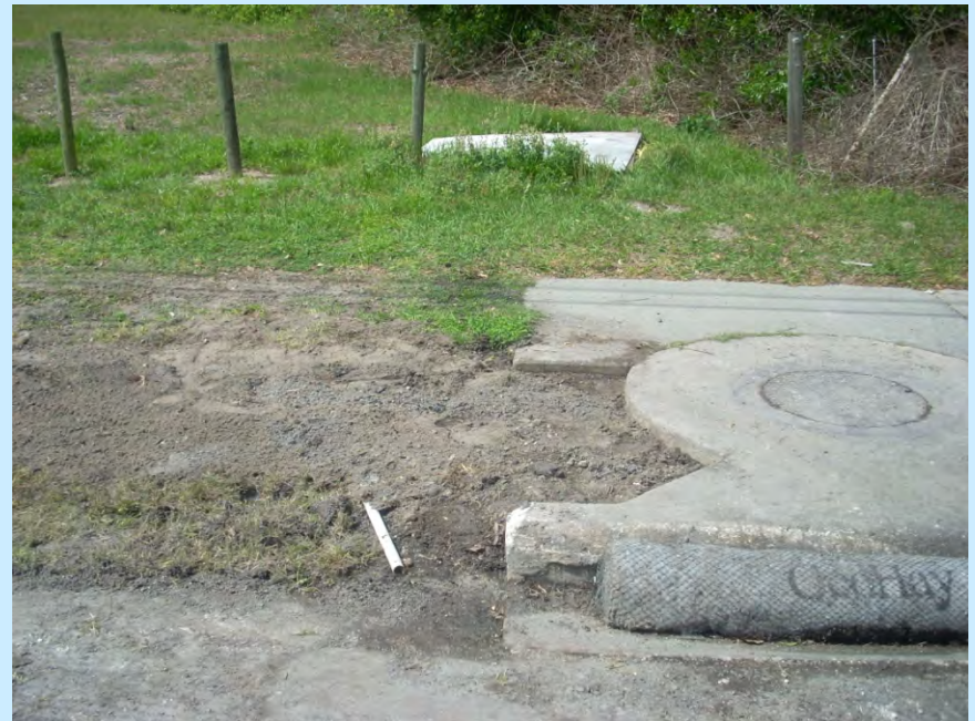
Unknown pipe to inlet
